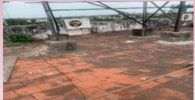
Damaged Weather proof Tiles on the terrace
