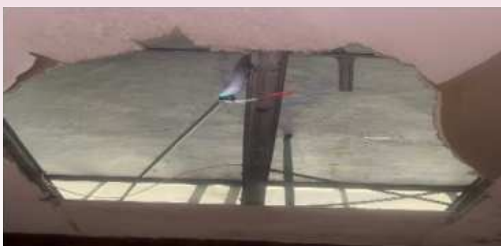
Crack formed in the ceiling
