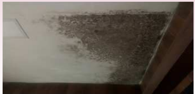
Damaged False roof due to water seepage
